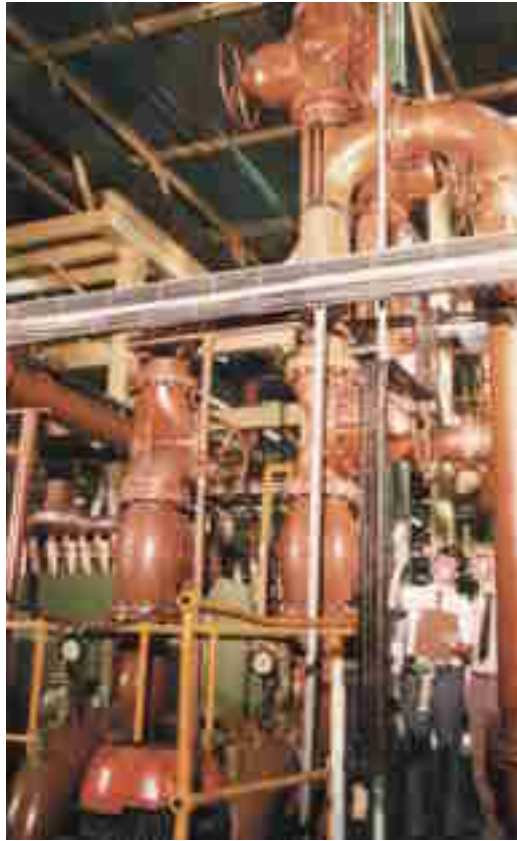
Large A Type valves installed in a distillery
